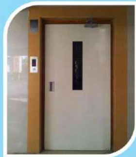
Channel with Swing Doors
